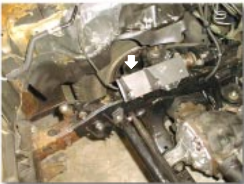
Photo #3 (Passenger side)
